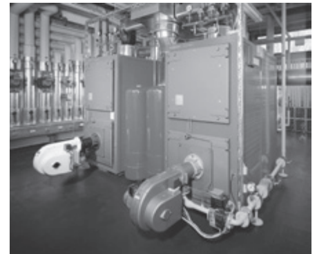
Gas inlet pressure monitoring on high-performance boilers
